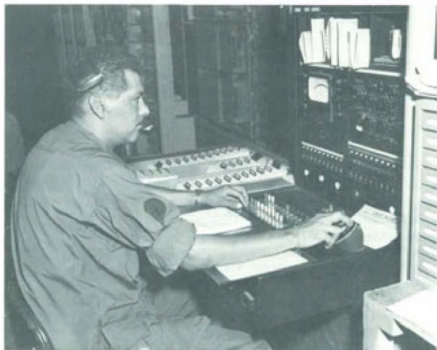
TEST BOARD IN ONE OF THE MANY DIAL TELEPHONE EXCHANGES IN VIETNAM
