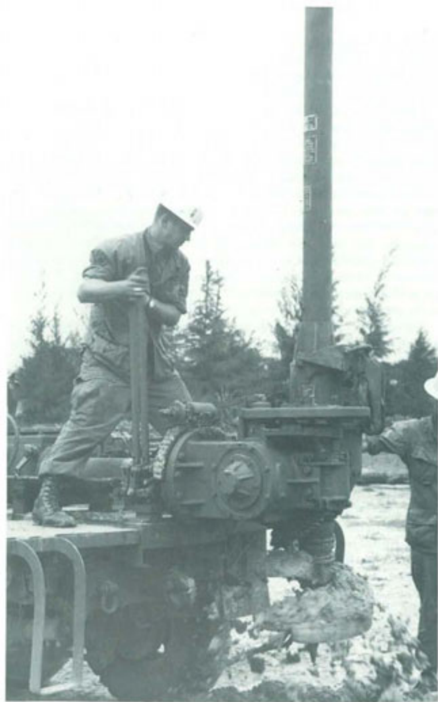
SIGNALMEN OPERATE A POSTHOLE DIGGER AT GHU LAI, where cable telephone poles are being installed.
